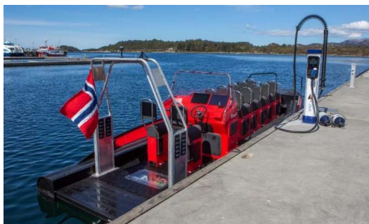
Fig. 59: EV charger deployed for small vessel charging according to Paper 11082
